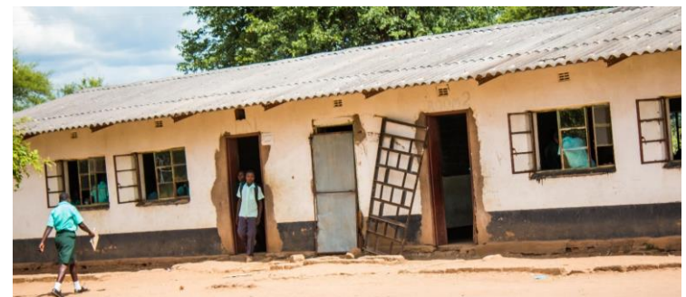
Hwata Secondary – March 2022, before repairs
